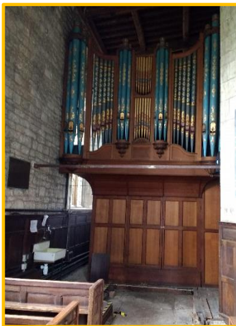
The area in front of the organ in St Andrew's Church has been cleared ready for the installation of toilet facilities.
